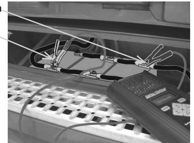
Battery Bank of 3 Batteries
